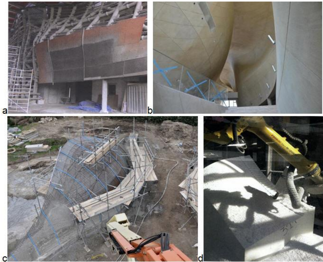
Figure 1. Modern technologies of constructing archy designs: a – non-removable formwork of waterproof plywood [1]; b – bent walls of the museum [1]; c – reinforcing cage for acoustic frames [2]; d – manufacture of polystyrene formwork [3]
